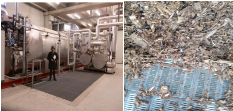
1 MW power plant component
